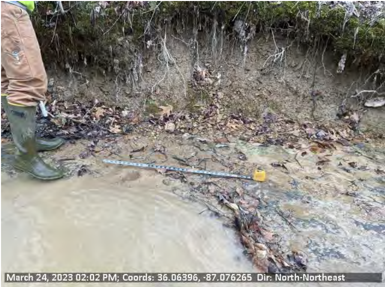
20 View of STR-6-I proposed sediment removal location on left descending bank measuring approximately 2'x1', and 0.25" deep.
