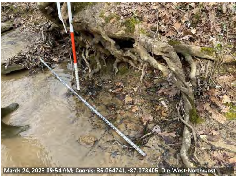
13 View of STR-6-B proposed sediment removal location under tree root on left descending bank, measuring approximately 4'x1', and 0.5" deep,
