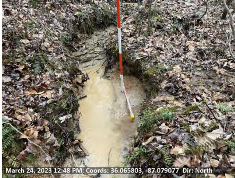
27 View of WWC-18-A proposed sediment removal location on left descending bank, measuring approximately 3'x1', and 3" deep.
