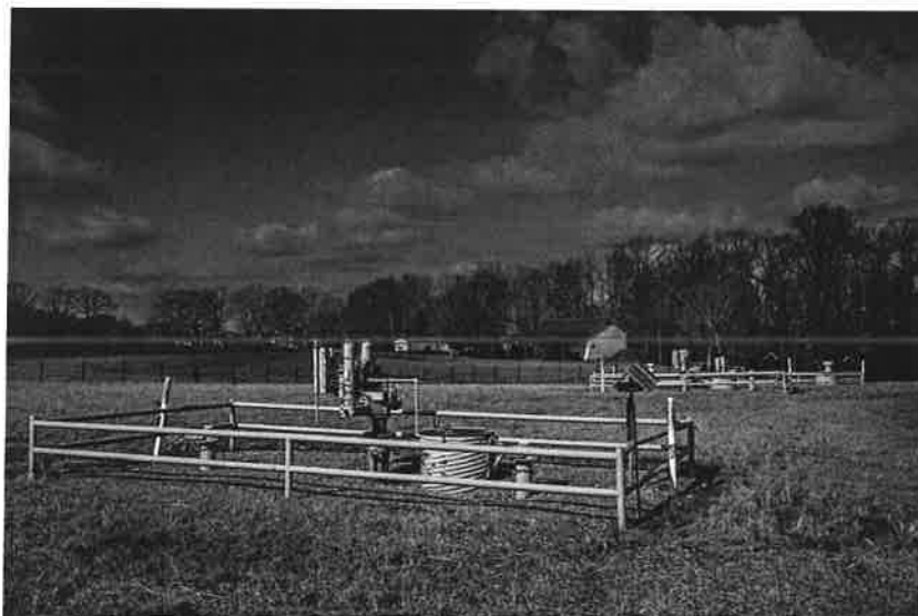
📷 A pumping station in Dickson County at the site of a 1992 gas line rupture. (Photo: John Partipilo)
